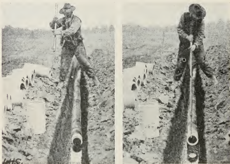
Fig. 12.—Laying small tile with a tile hook from the top of the trench. (Courtesy of International Harvester Co.)
